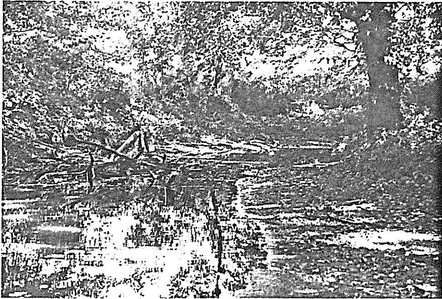
Scour Channel at the North End of the Pasture
